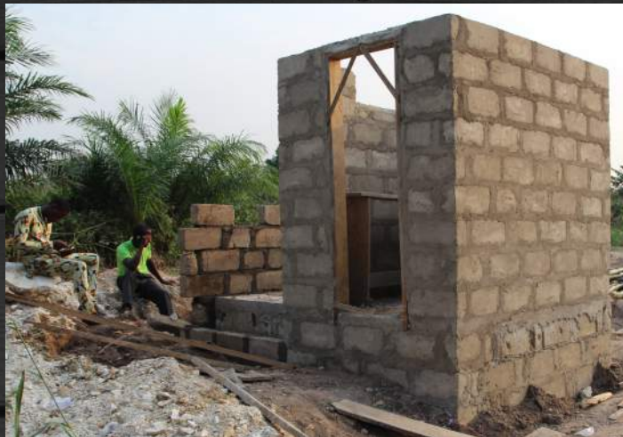
This is the bathroom door frame on the right, with a storage room entrance on the opposite side.
